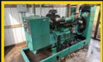
1990 Cummins Onan 125 KW Genset - Salem, IN
