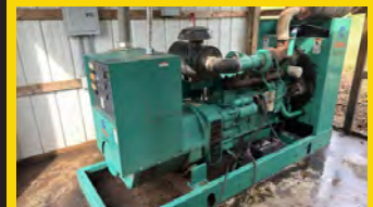
1990 Cummins Onan 125 KW Genset - Salem, IN
