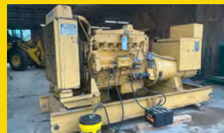
Caterpillar 3406 260 kW Skid-Mounted Diesel Generator Set Piketon, OH
