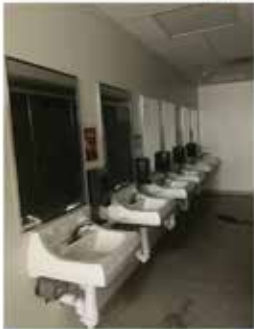
Sinks with Motion Controlled Faucets Sink Measures 10"x20"x18" Includes Sloan Motion Sensor Faucet & Mixing Valve $50.00 Each 12 Available
