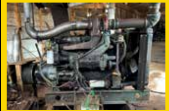
Detroit 671 Power Unit
