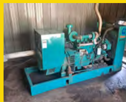
1996 Onan Cummins Genset Ickesburg, PA
