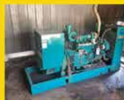
1996 Onan Cummins Genset Ickesburg, PA
