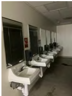
Sinks with Motion Controlled Faucets Sink Measures 10"x20"x18" Includes Sloan Motion Sensor Faucet & Mixing Valve $50.00 Each 12 Available
