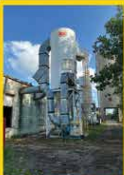
MAC & Dynacom Industrial Dust Collection System
