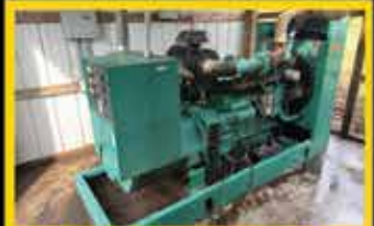
1990 Cummins Onan 125 KW Genset - Salem, IN
