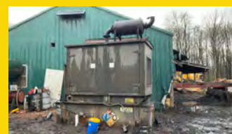
Caterpillar 175 KW Genset
