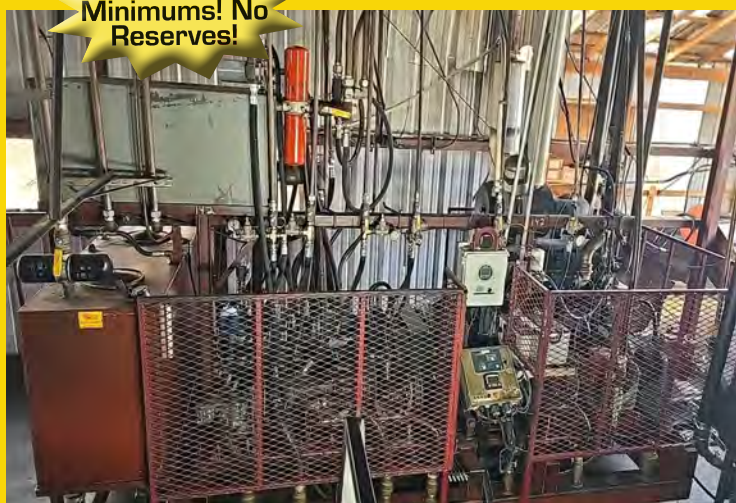
2009 Iveco Power Unit and Hydraulic Pack
