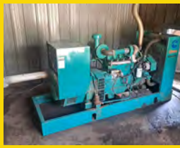
1996 Onan Cummins Genset Ickesburg, PA
