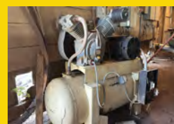
Ingersoll Rand 7100 Air Compressor
