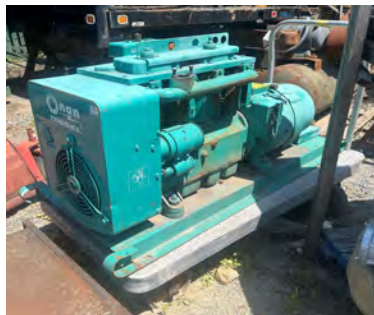
Onan Diesel Generator 12 KW 3 Phase
