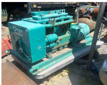
Onan Diesel Generator 12 KW 3 Phase
