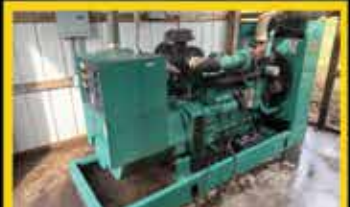
1990 Cummins Onan 125 KW Genset - Salem, IN
