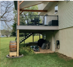
Deck and steps with roof. Exposed Douglas fir beams with standing seam roof
