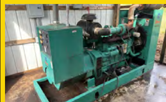
1990 Cummins Onan 125 KW Genset - Salem, IN
